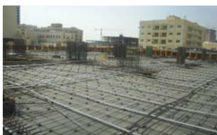
PBL has marked its post tensioning systems globally. Tendon installation in the Middle East.
